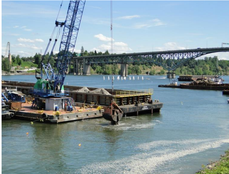
Chemical isolation layer sand placed in 1-foot lifts using traditional clamshell bucket.
